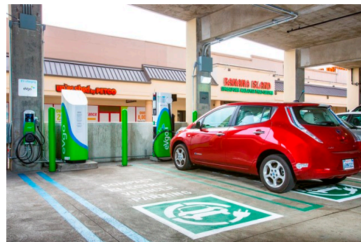
Figure 3: A set of EV charging stations at the Westlake Shopping Center in Daly City
